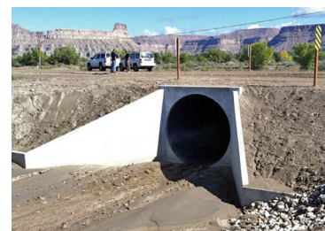
To prevent flooding and erosion this culvert was replaced with a larger culvert and additional wingwalls.
