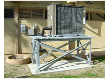
An elevated heat pump is an example of elevating equipment to prevent flooding damage.
