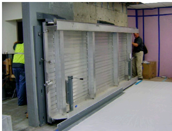
A flood door is an example of dry floodproofing a building.
